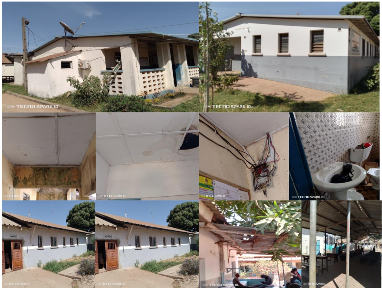
Figure 3: Structural Defects identified in Brikama District Hospital
