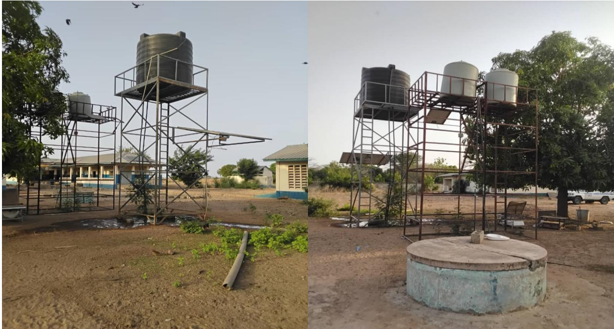
Figure 13. Overhead water tanks for solar powered borehole in the health facility
