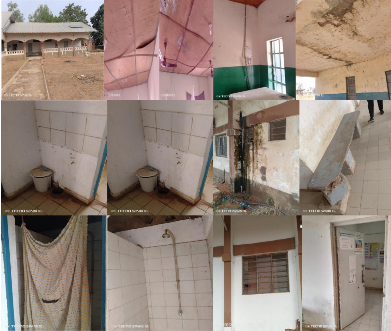
Figure 4. Structural Defects identified at Chamen Health Center
