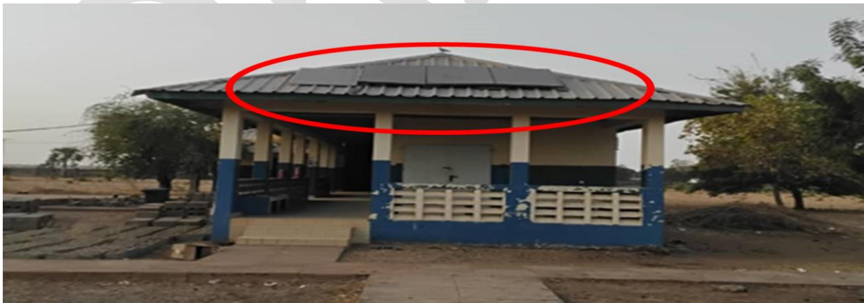
Figure 14. Solar PV System at Chamen Health Facility
